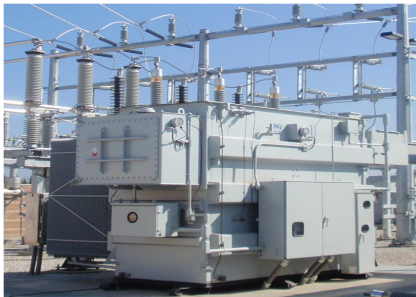
Typical Power Transformer
