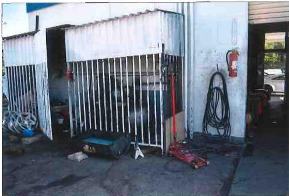
#8 Enclosure with the compressor.
