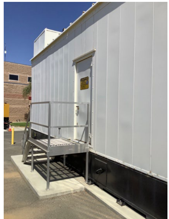
Photo 12: Layer 2 - Generators near the main gate are properly enclosed.
