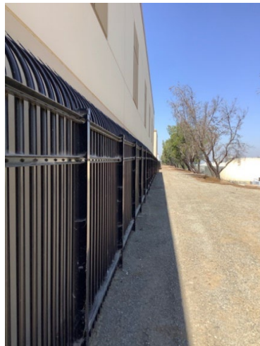
Photo 3: Layer 1 - The fencing on the south side shown here is easily defeated by entering via the nearby buildings, which are not owned or controlled by RWQCP.
