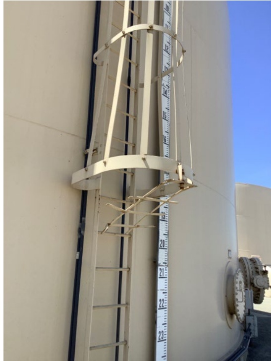
Photo 13: Layer 2 - Tank ladder is insecure.
