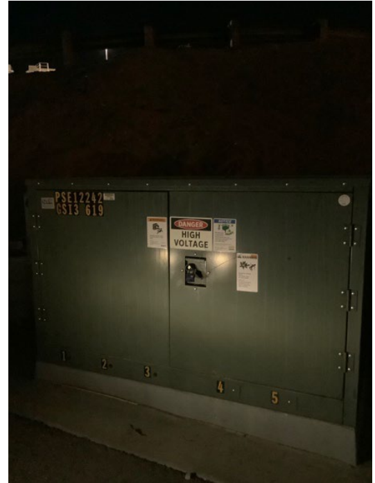
Photo 16: Layer 2 - These transformers are padlocked, although not caged. This is effective.
