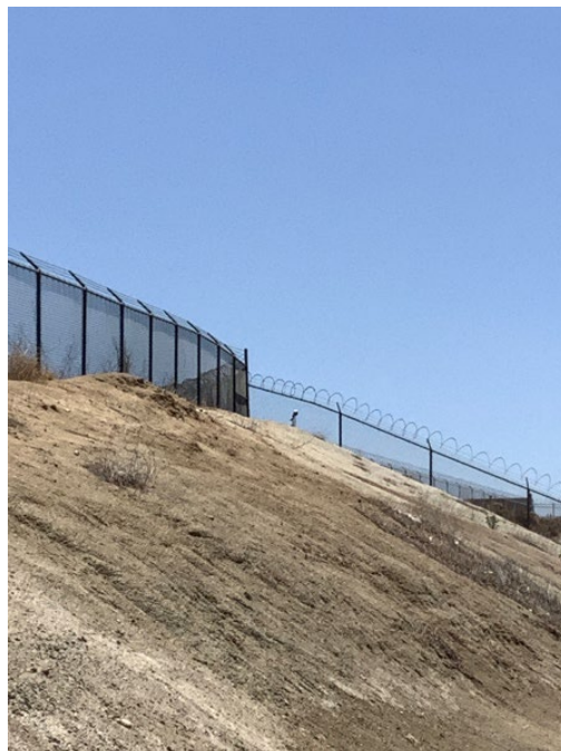
Photo 11: Layer 1 - Fencing around the east perimeter does not match the very strong fencing elsewhere. The razor wire helps, however the fence itself is low (6-ft) and can be cut. There is no effective alarming in the area.
