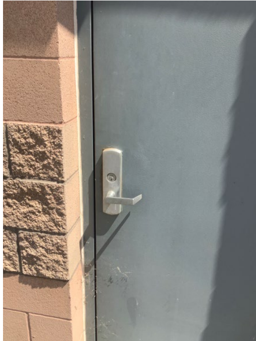
Photo 17: Layer 3 - Typical process area door. Metal in metal frame, however this door has no astragal.
