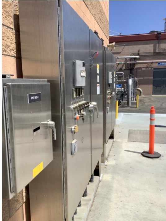
Photo 25: Layer 5 - Exterior accessible panels should be locked.
