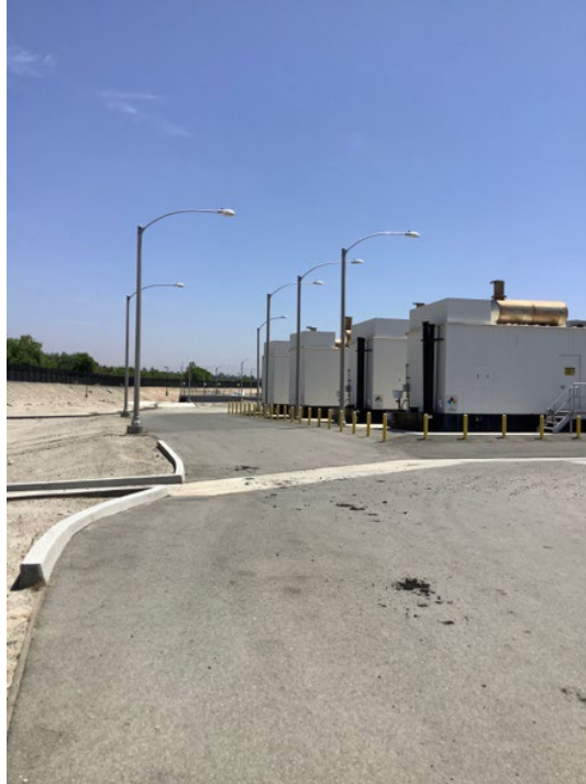
Photo 15: Layer 2 - Effective lighting at the north generators.
