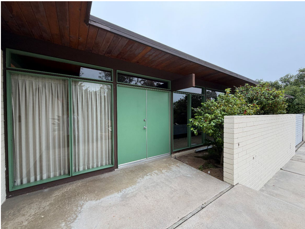
Figure 4 – Edie façade fenestration, eave, and roof beams behind freestanding garden wall, view southwest
