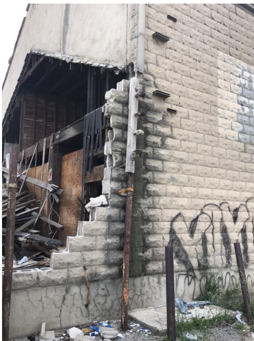
Soda Works Building: Source G T Loudon AIA Photography, February 2022 ; Figure # D-14 View east of partially remaining west façade and exposed interior showing prior damage by fire.
