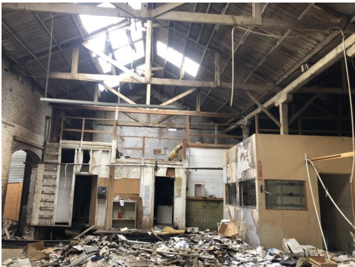
Barley Mills Building Interior: Source G T Louden AIA Photography, February 2022; View to south façade of original 1891 structure; note the fire damaged wood floor and joists in near foreground; added mezzanine and interior wood framed enclosed space; note wood roof trusses viewed at location at centerline of the two gables; Figure # D-17
