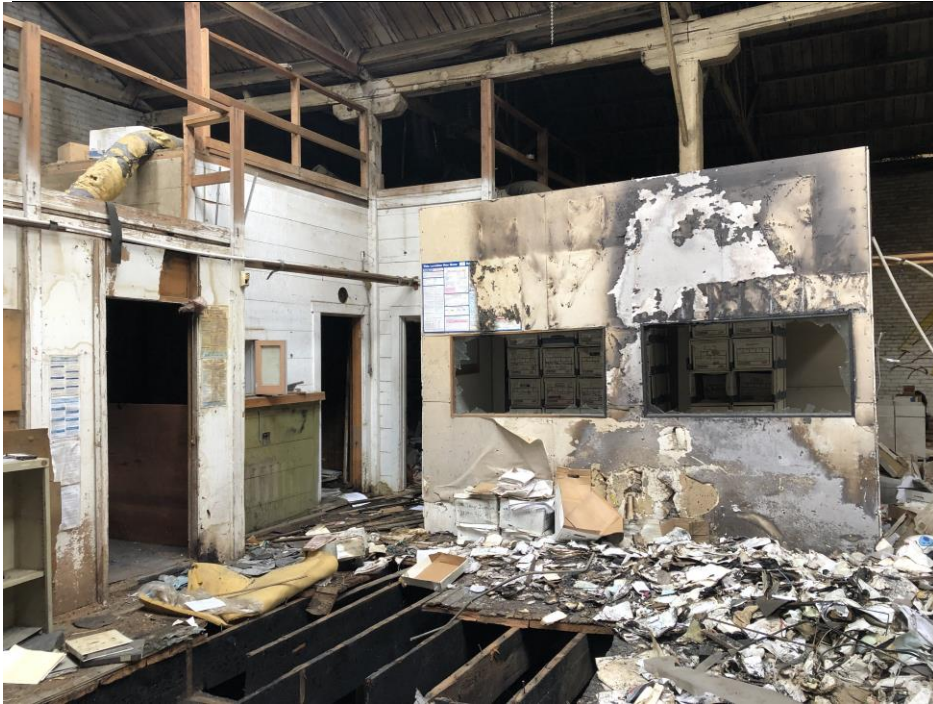
Barley Mills Building Interior: Source G T Louden AIA Photography, February 2022; View to southwest corner of original 1891 structure; note the fire damaged wood floor and joists in near foreground; added mezzanine and interior wood framed enclosed space; Figure # D-16
