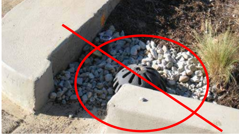
Figure 6: Incorrect Placement of an Overflow Inlet.
