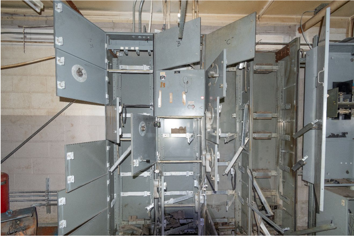
Figure 27 - Electrical system damage
