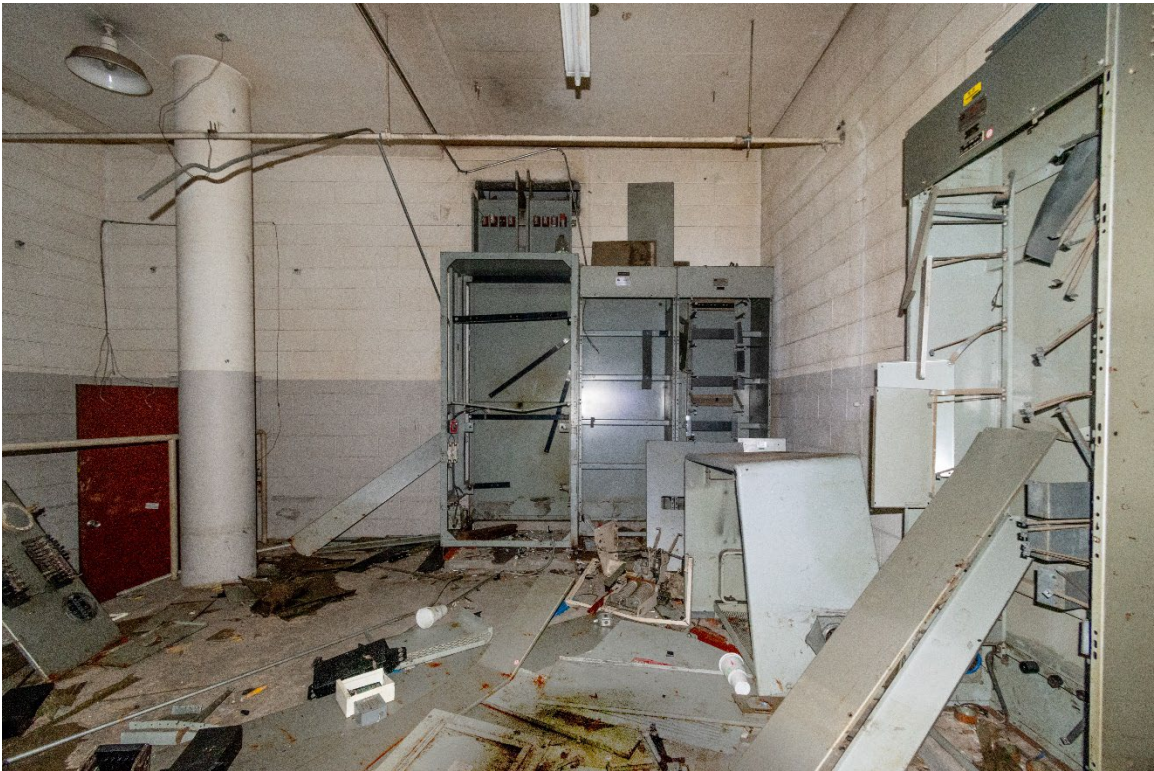
Figure 28 - Electrical system damage
