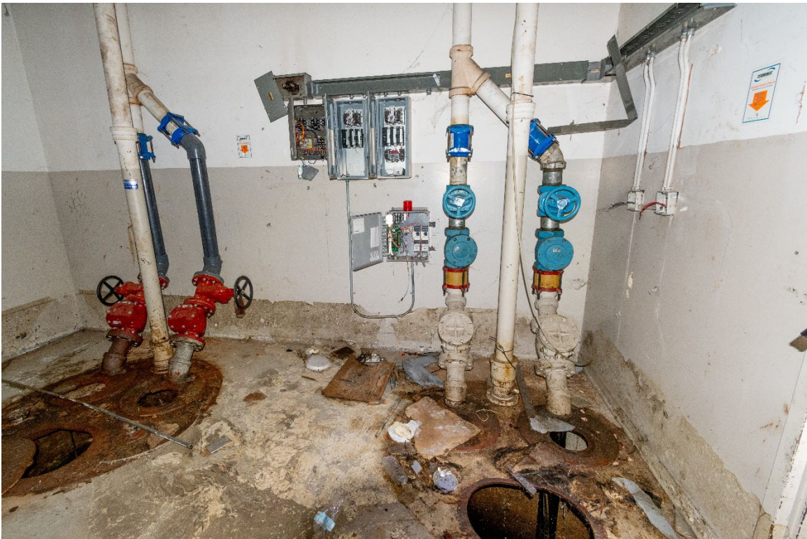
Figure 26 - Plumbing system damage
