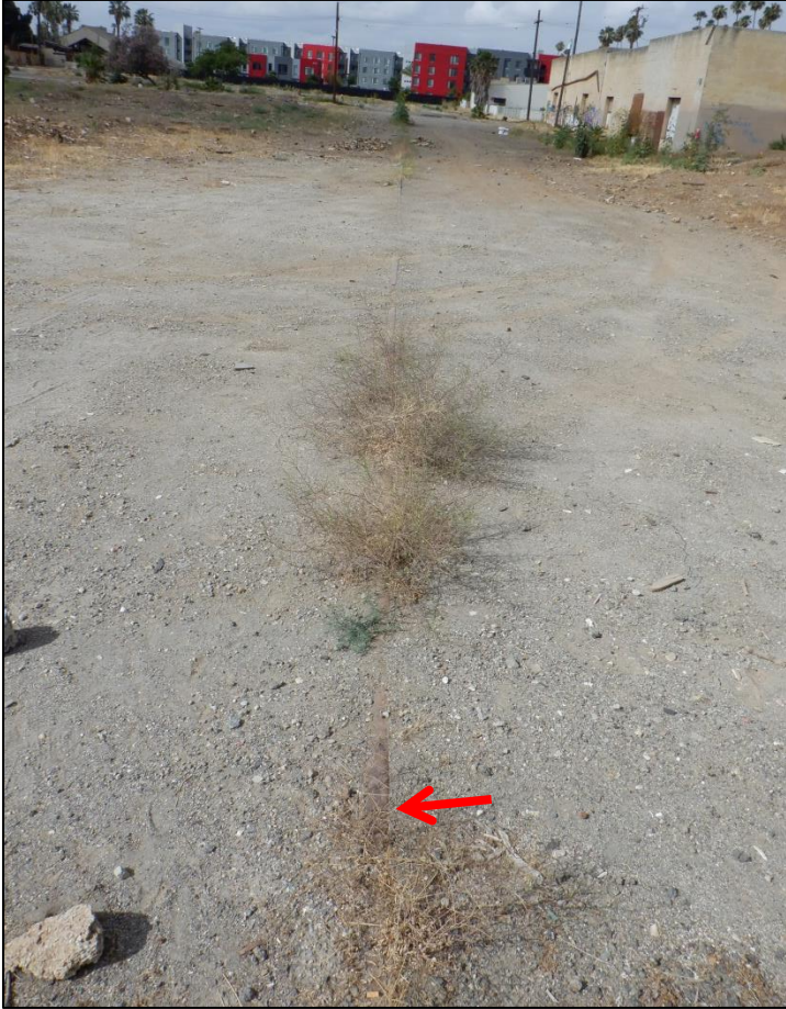
Figure 15. Partially exposed rail east of 3596 Commerce Street, facing south
