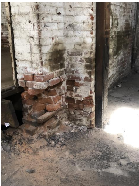
Barley Mills Building Interior: Source G T Loudon AIA Photography, March 2022; Interior view of south east façade, near the corner; note the brick masonry foundations have failed at the original west façade opening at the former exterior doorway jamb; Figure # D-21.
