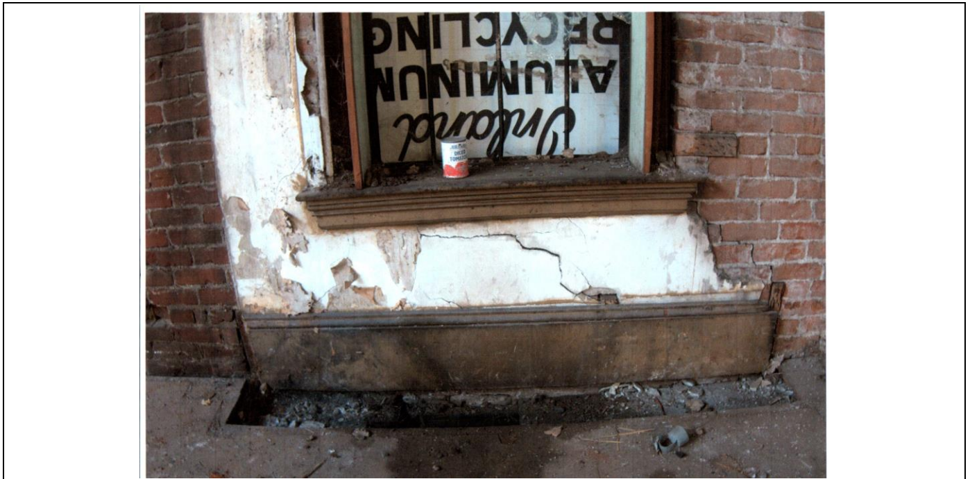
Figure # 20: The remaining original south façade interior wood window trim details at the named "office" area of the Barley Mills Structure: wall base and trim cap; window apron, window sill, window jamb trim/sash window weight box. See Appendix D.
