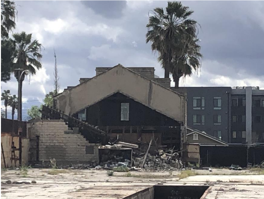
Soda Works Building: Source G T Loudon AIA Photography, February 2022 ; Figure # D-13 View south of partially remaining north façade and roof collapse from previous fire damage.
