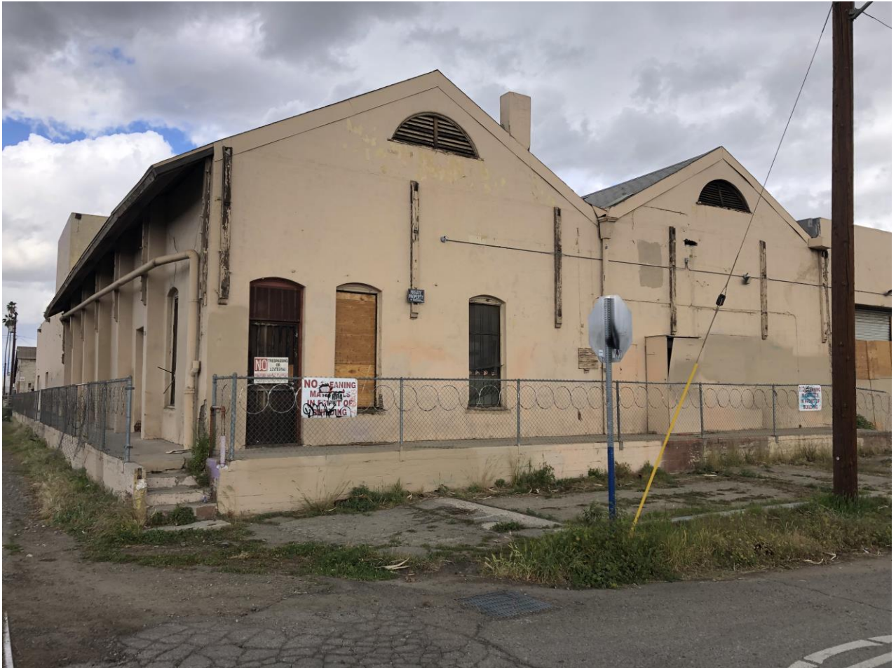
Figure # 22: Existing site context, photograph dated 2022; south façade of the Barley Mills Building and the original wood framing supports for the original canopy at south gable and at west façade. Existing chimney at southeast gable is not visible in the 1906 era photograph. This chimney is not proposed for retention without structural retrofitting.
