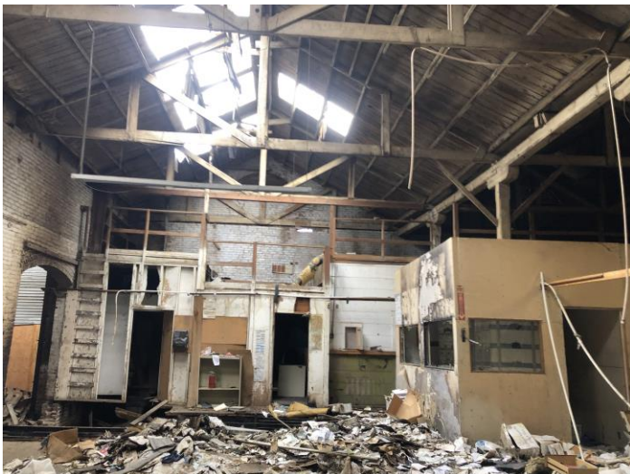
Barley Mills Building Interior: Source G T Loudon AIA Photography, February 2022; View to south façade of original 1891 structure; note the fire damaged wood floor and joists in near foreground; added mezzanine and interior wood framed enclosed space; note wood roof trusses viewed at location at centerline of the two gables; Figure # D-17
