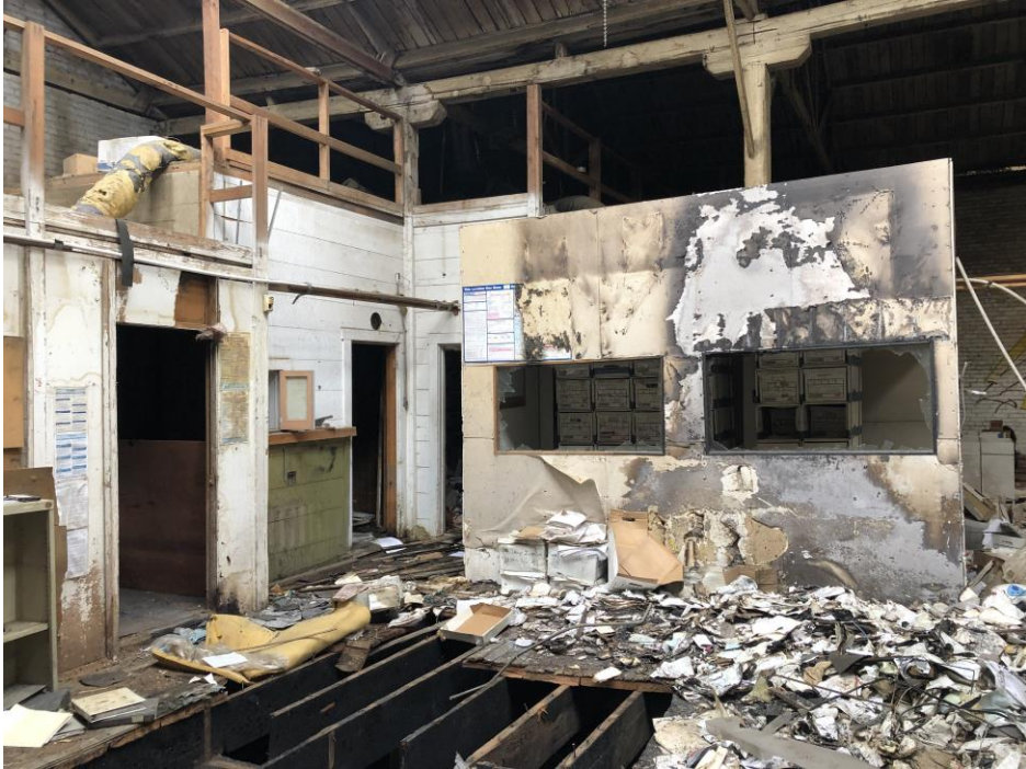
Barley Mills Building Interior: Source G T Loudon AIA Photography, February 2022; View to southwest corner of original 1891 structure; note the fire damaged wood floor and joists in near foreground; added mezzanine and interior wood framed enclosed space; Figure # D-16
