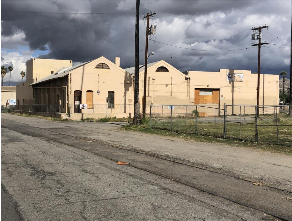
Barley Mills Building: Source G T Louden AIA Photography, February 2022; Southwest corner overview and railroad siding in Commerce Street; Figure # D-11
