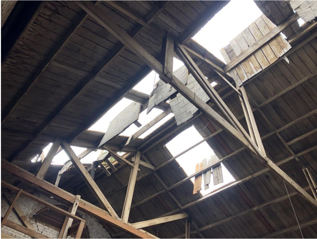
Barley Mills Building Interior: Source G T Loudon AIA Photography, February 2022; View of wood roof framing, board finish at the joists; the south wall brick façade and the half circular vent; the roof openings for skylights are not original and are not proposed to be restored. Figure # D-18
