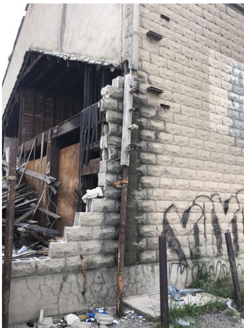
Soda Works Building: Source G T Loudon AIA Photography, February 2022 ; Figure # D-14 View east of partially remaining west façade and exposed interior showing prior damage by fire.
