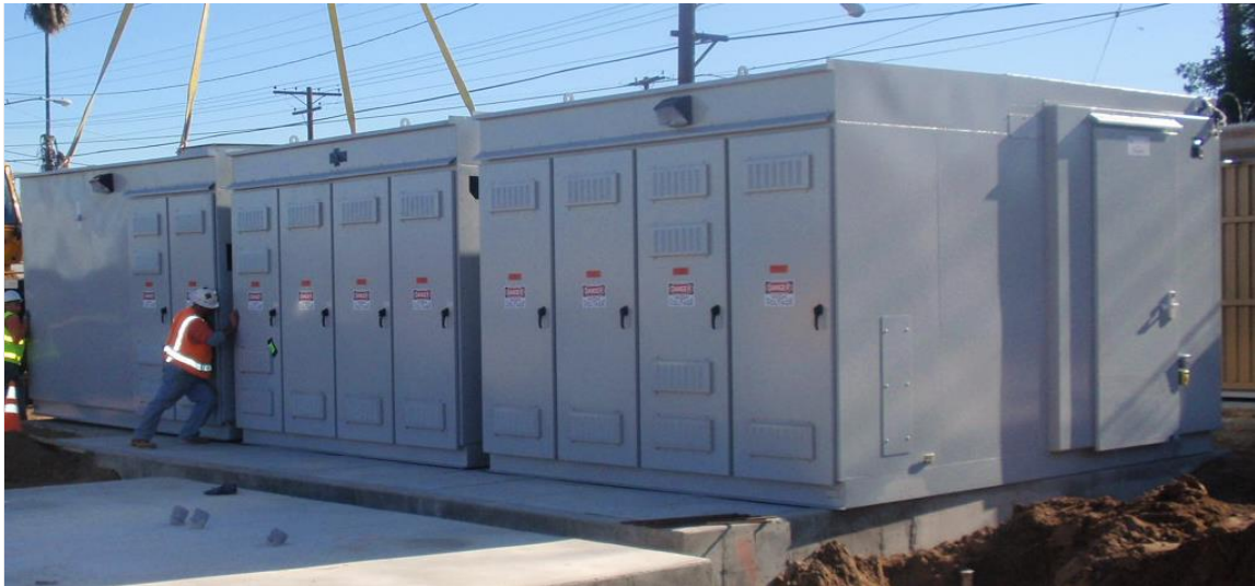
Typical 15KV Metalclad Switchgear
