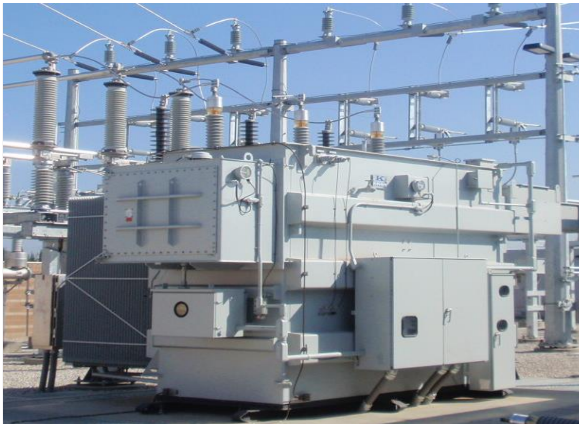
Typical 69KV Power Transformer
