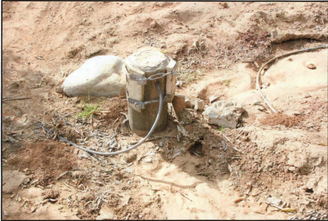
Another example of standpipe irrigation head (Close-up)
