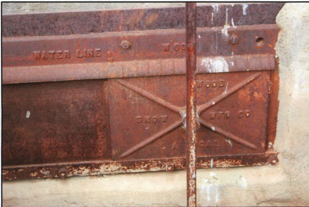
Gate valves within the large standpipe feature (Detail)
