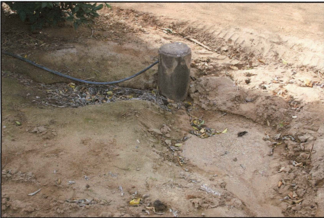
Example of low-profile standpipe irrigation head; these are placed along South-eastern (upslope) edge of the orchard and across the middle (Close-up)
