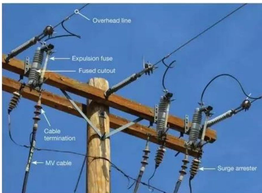
Fused Cutouts on Crossarm
