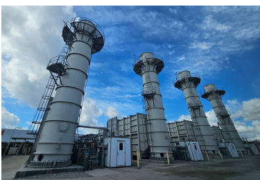
Springs Power Plant (36MW)
