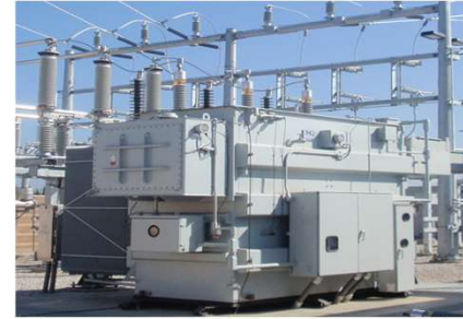
Typical Substation Transformer
