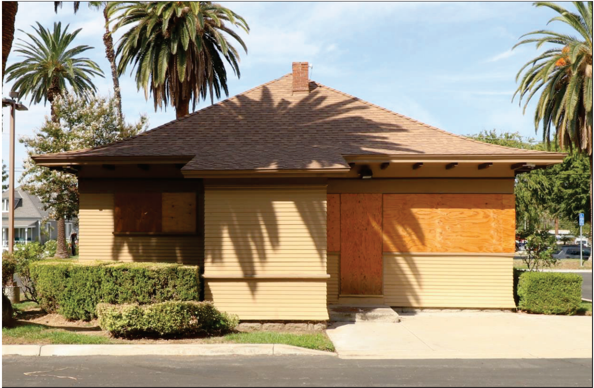
Photo 4. East elevation, view west (10/7/24). Fire damage was not evident on this rear elevation.
