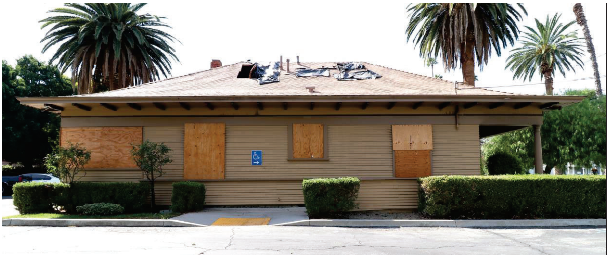
Photo 5. North elevation, view south (10/7/24). Note holes in the roof and minor evidence of fire under the eaves.
