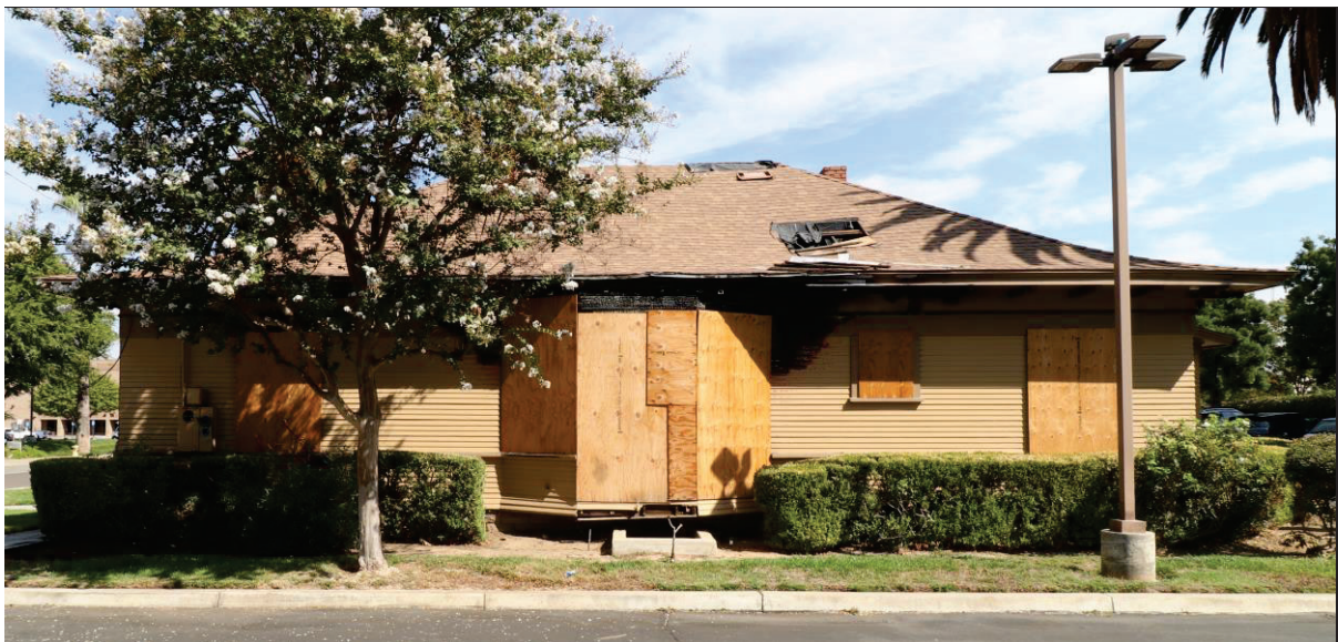
Photo 3. South elevation, view north (10/7/24). Note holes in the roof and charring along the eave and bay window.
