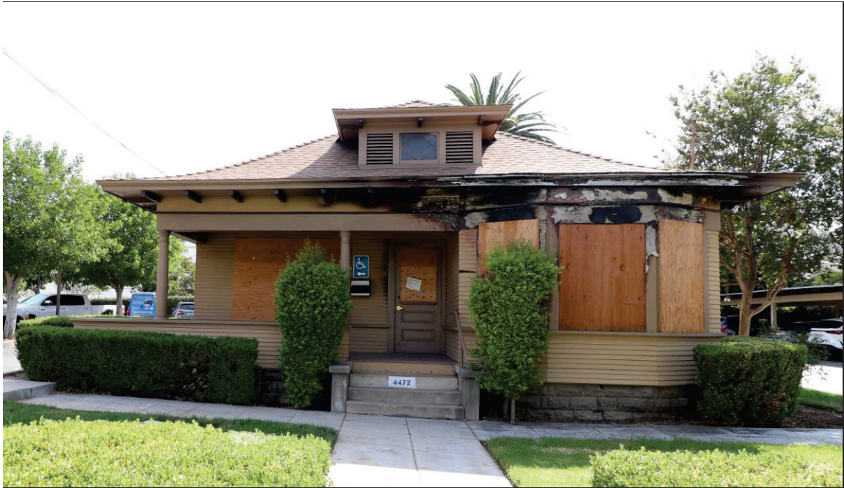
Photo 2. Façade, view east (10/7/24). Note fire damage above the porch and bay window.
