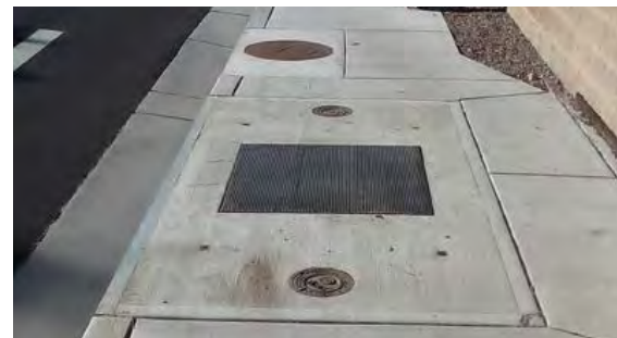
Figure 2b. Filterra with Full Grate Photo
