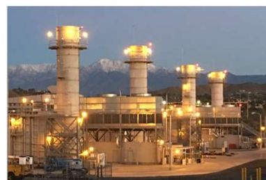
Riverside Energy Resource Center (RERC) (196 MW)
