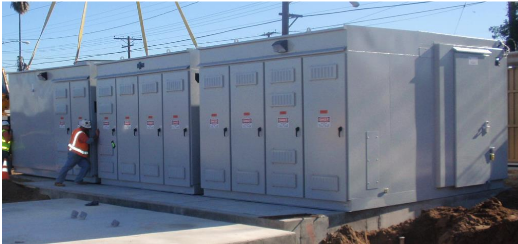
Typical Modern 15KV Metalclad Switchgear
