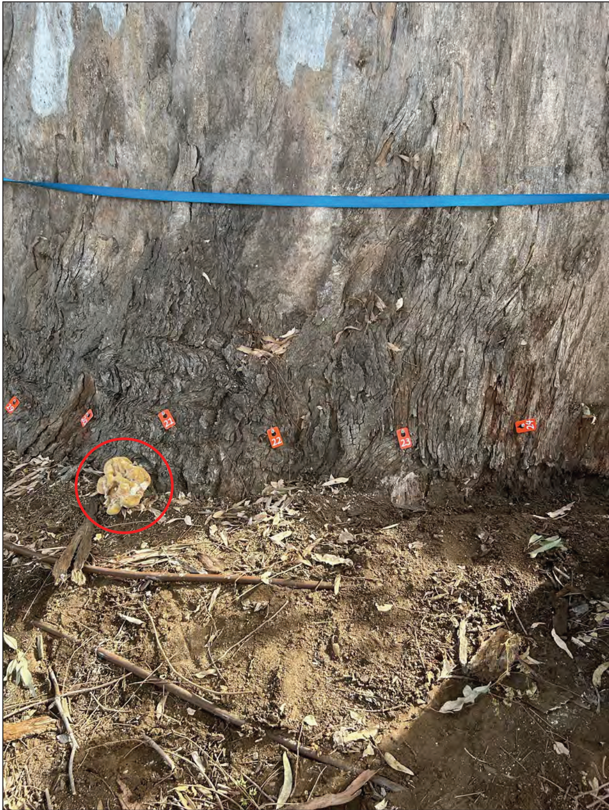
Figure 8: Drilling points 19 - 24 and a fungal conk.
