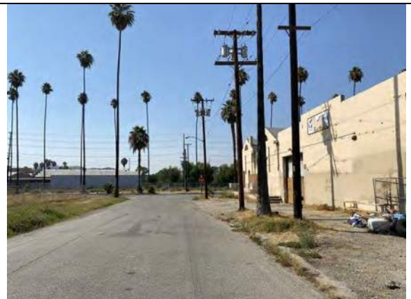
View of pole mount transformer
