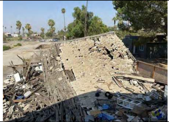
View of the portion of the building collapsed due to recent fire
